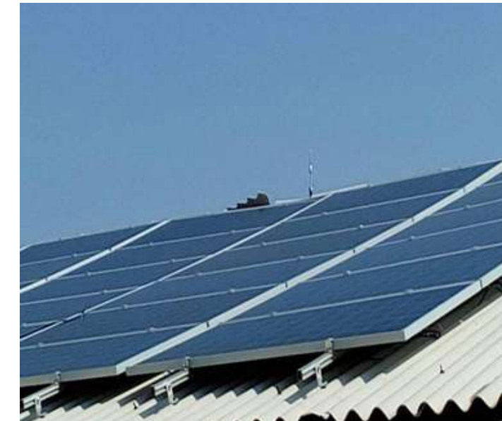
Heliacal Power (KR) - 6.5 MWp
