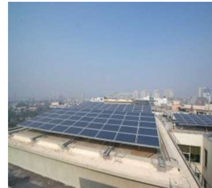
Chimes Group - 450 KWp
