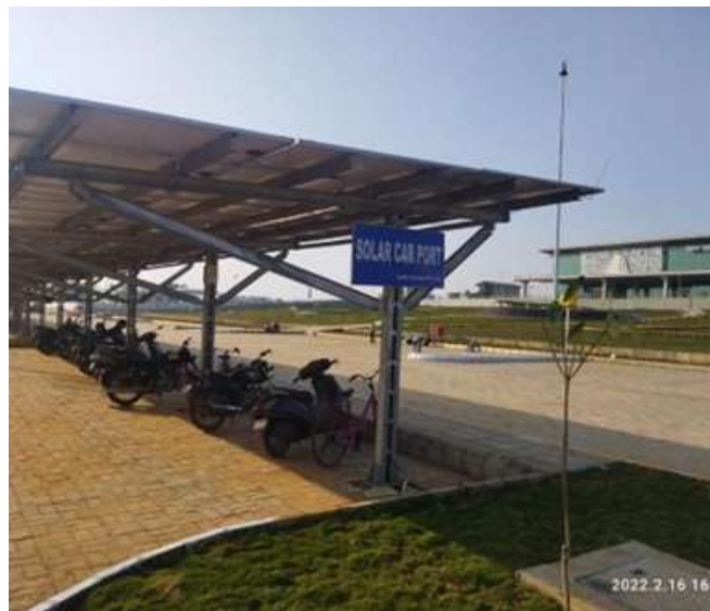
Deoghar Airport (JH.) - 385 KWp
