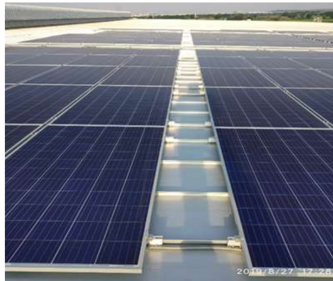
Amazon India (HR) - 500 KWp
