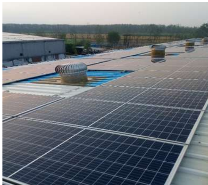
Ganesh Ecotech (TS) - 3 MWp
