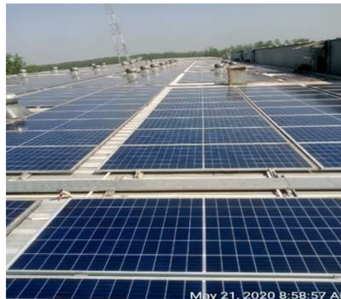
Ganesh Ecopet (TS) - 2 MWp
