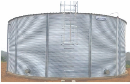
Fire / Drinking Water Storage Tank
