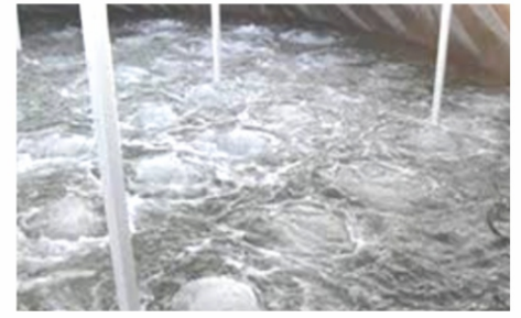
STP Aeration Tank
