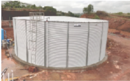
Raw Water Tank
