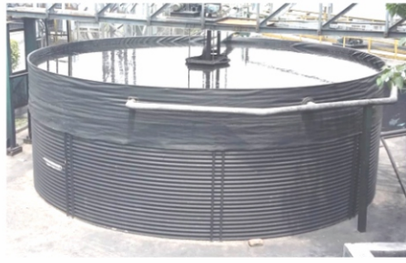
ETP Clarifier Tank
