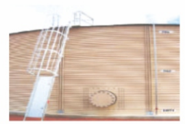
Safety Caged Ladder, Manway & True Level Indicator
