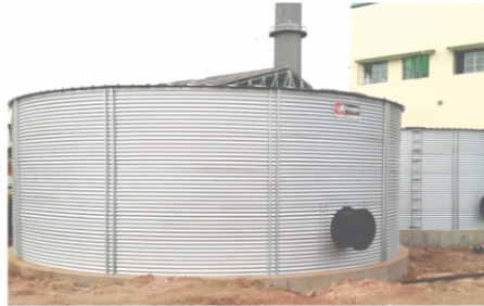
DM Water Tank
